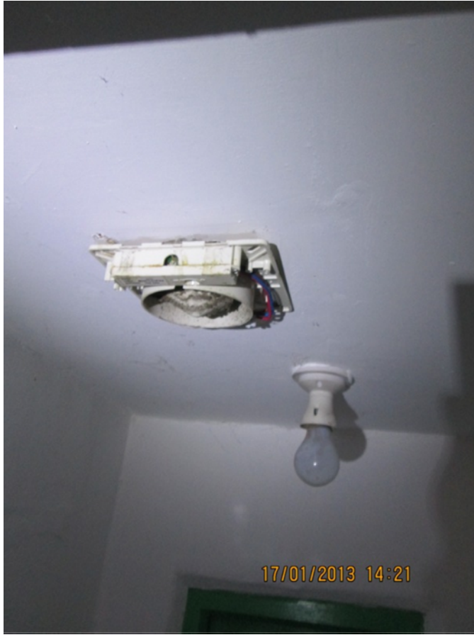
11) Damage ventilation fan exposing live electrical connections.
